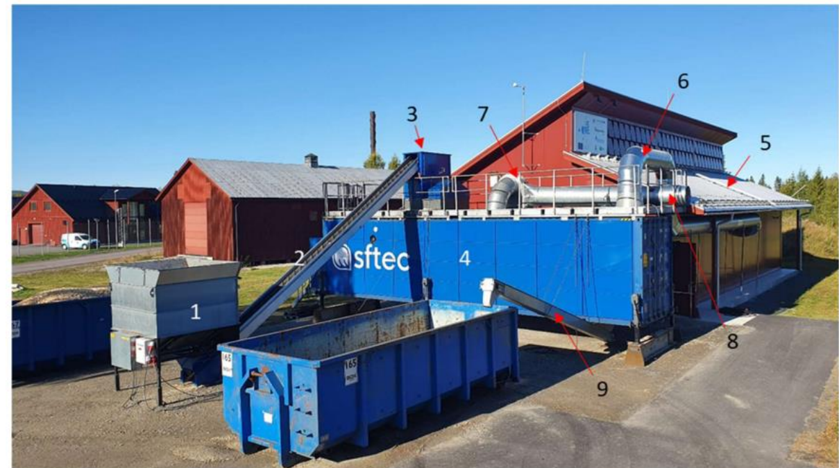
Figure 5, the layout of biomass drying test setup where the ModHeat® dryer is installed to the testing site BTDC (Boden, Sweden).
